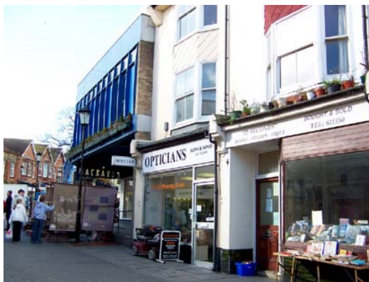
Deteriorating and poorly maintained shop fronts
