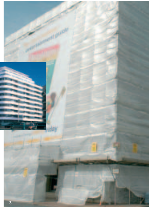
Embassy Court - 1. Dilapidated and unloved 2. How it will look after restoration 3. As it looks today
